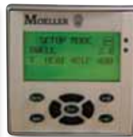
Simple control panel
